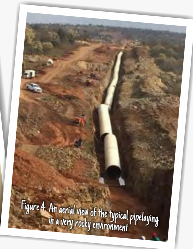
Figure 3: Typical siphon section of pipe being laid and welders welding the pipes together.
